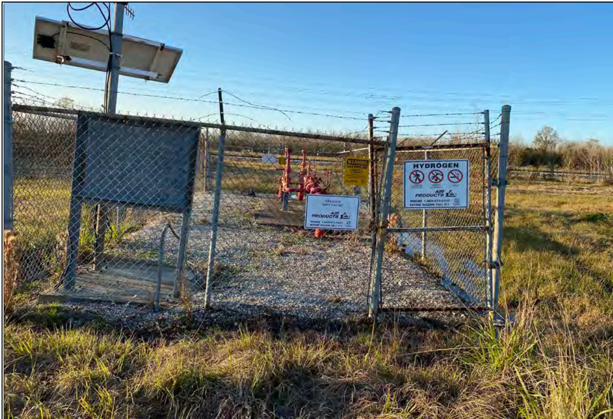
View of pipeline just outside the property boundary in the northwest corner, facing north.
