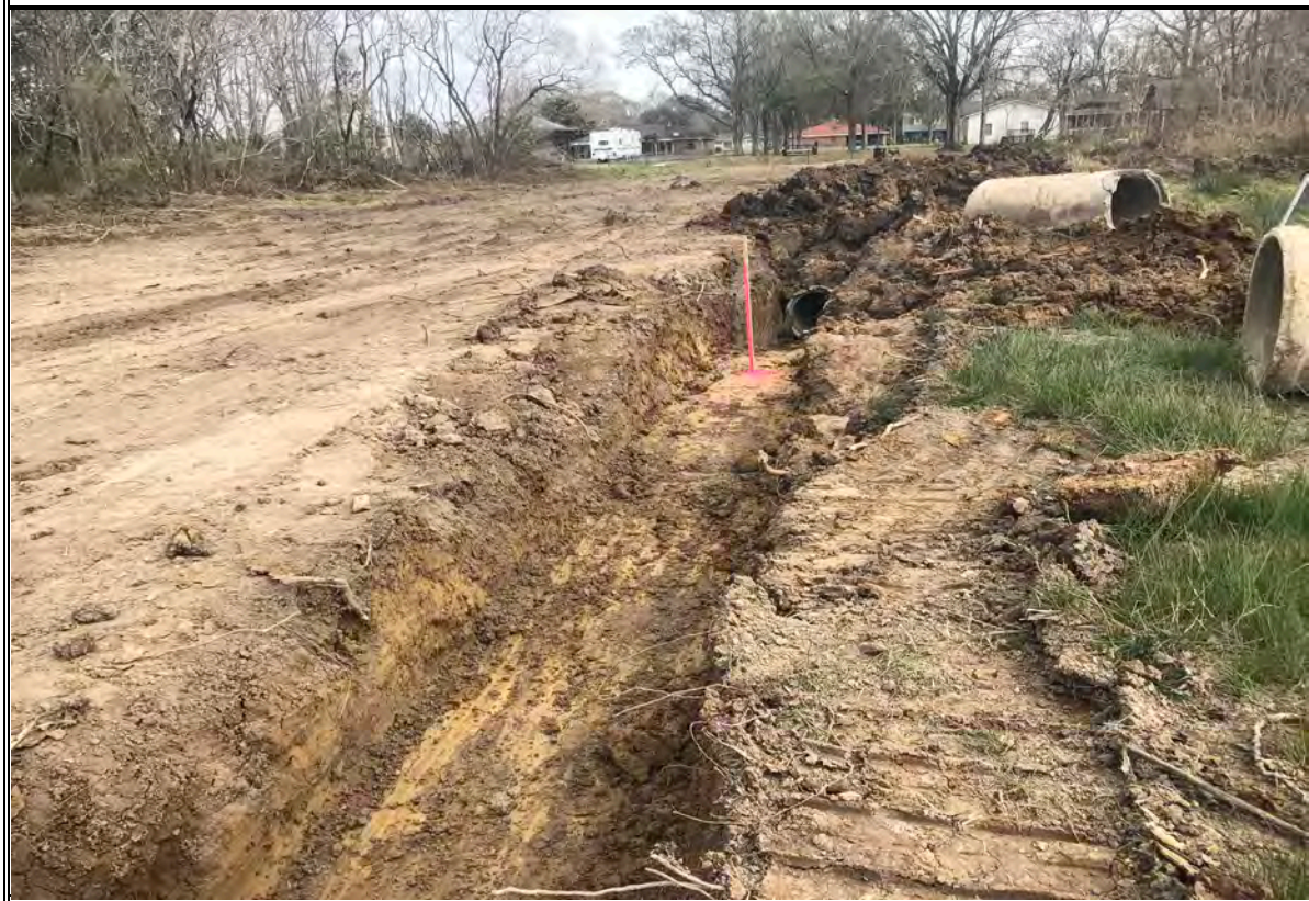
View of culvert additions being placed on property, perpendicular to A3A drainage ditch, facing east.
